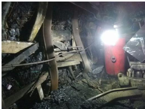
Bottom distortion of U-shaped steel
