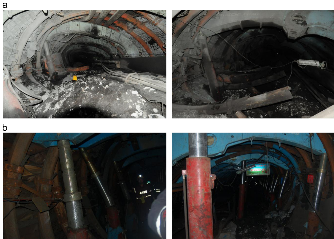
Fig. 10. Photographs of gateway damage taken after rock bursts occurring on (a) 11 August 2010, and (b) 1 March 2011.
